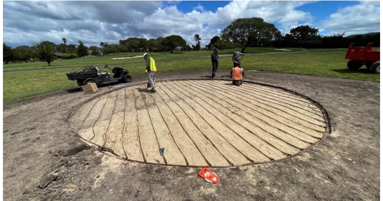
Figure 1. Typical round, island tee with drip tubing 12-inches apart. Tubing was buried 6-inches deep and then sodded.
