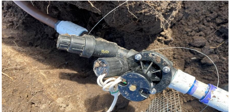
Figure 2. Example of an electric valve and combination filter and pressure regulator connected to a pre-made header line (left) and mainline (right).
